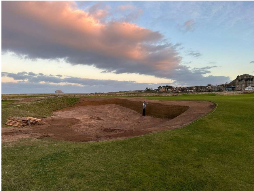
Figure 2: Scott in the renovated bunker on Redan showing the scale of the job.
