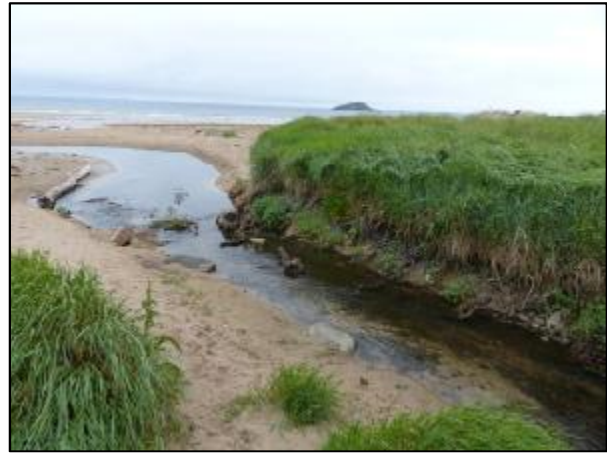
Under cutting and destabilisation of the gabions through the mouth of the burn
