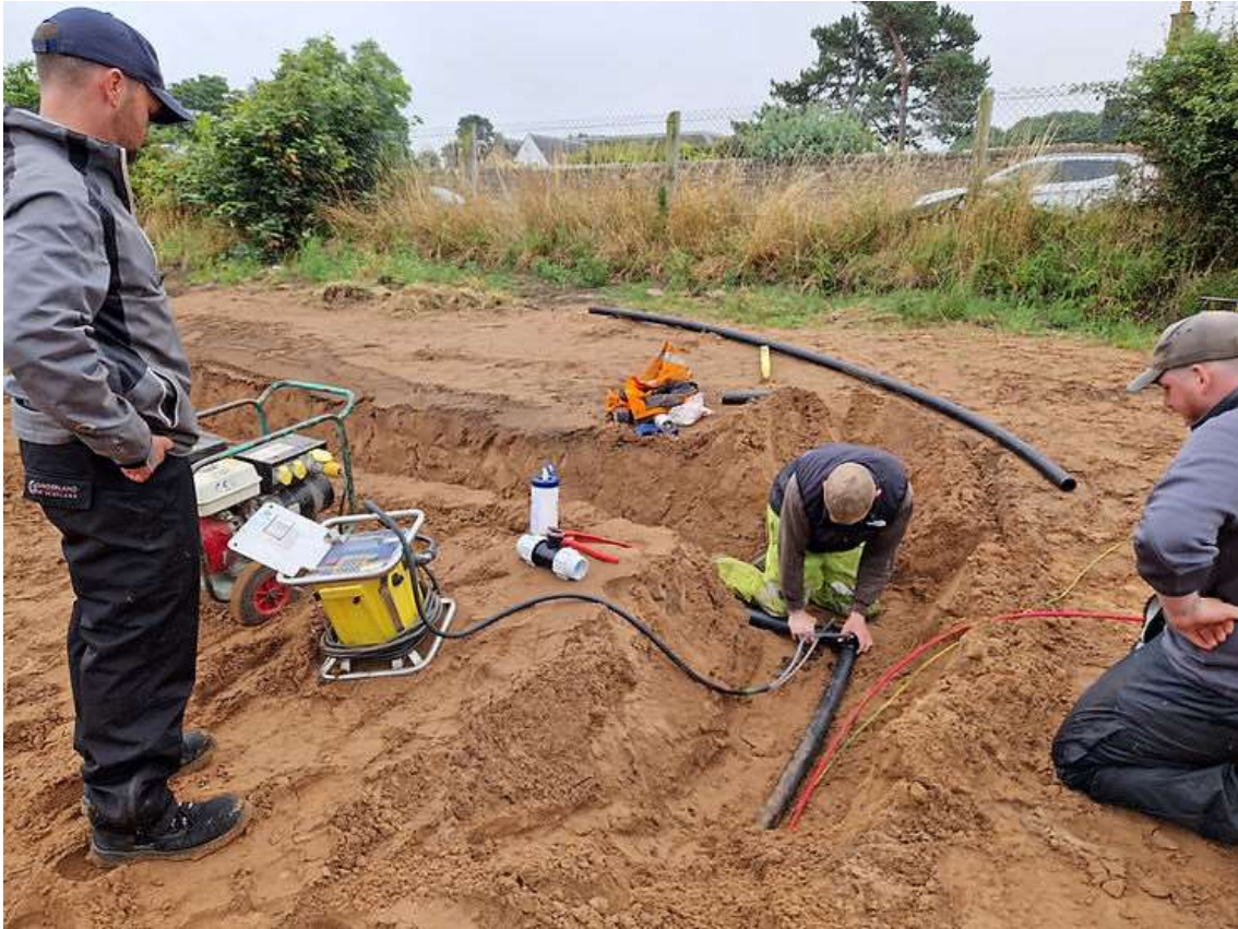
Graeme and Alex learning how to fusion weld pipe together by Dougie
