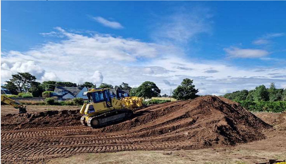
Scott in the Bulldozer starts to pile up the material to be screened.
