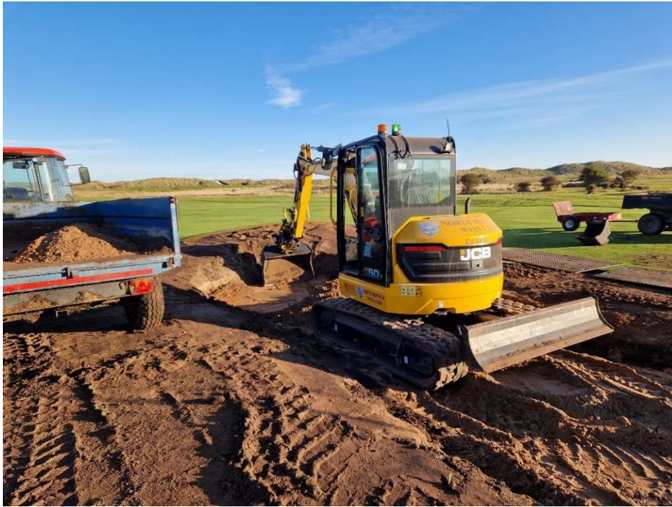
Figure 3: The digger excavating the old sand and revetted wall out before shaping.
