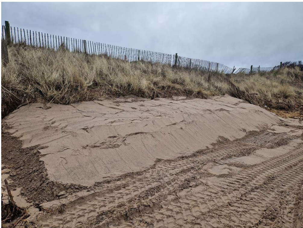
Figure 2: The same area as Figure 1 is built up with sand to increase the protection of the sandbags. This work will be continued along the entire protection area.
