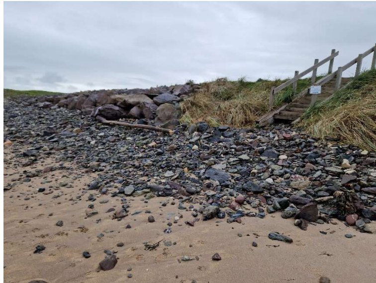
Figure 3: Burst rock-filled gabions beside the Rock Armoury at the 2 nd .
