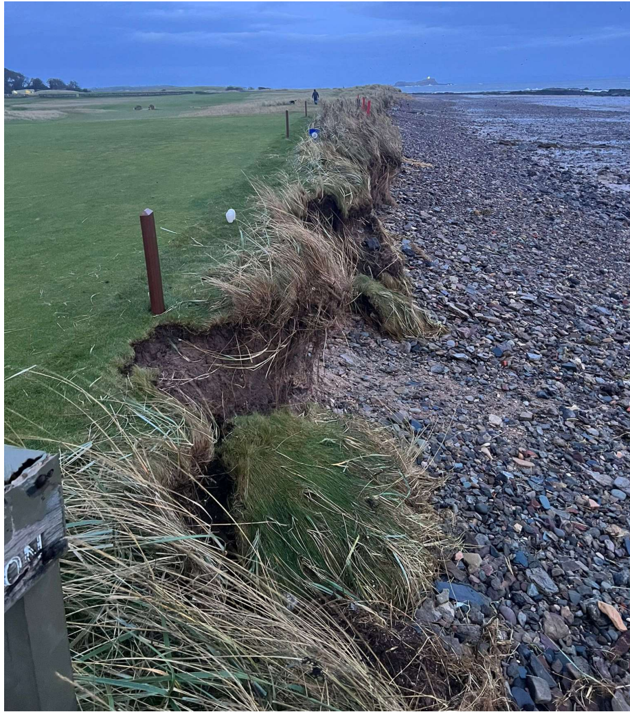
Figure 9: The damage at the 3 rd tees with a lot of the dune disappearing and been swept to sea.
