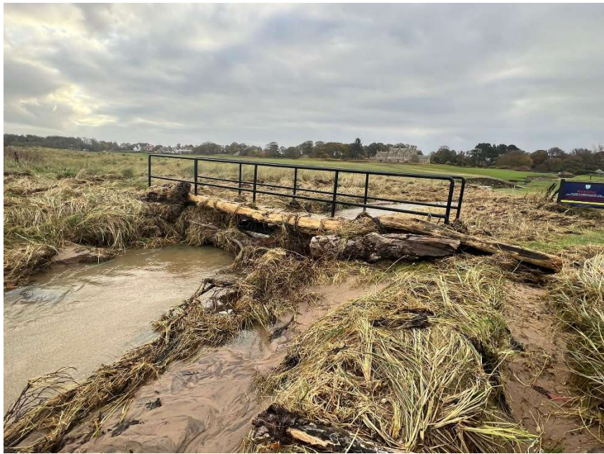
Figure 8: Debris obstructing the Eel Burn.
