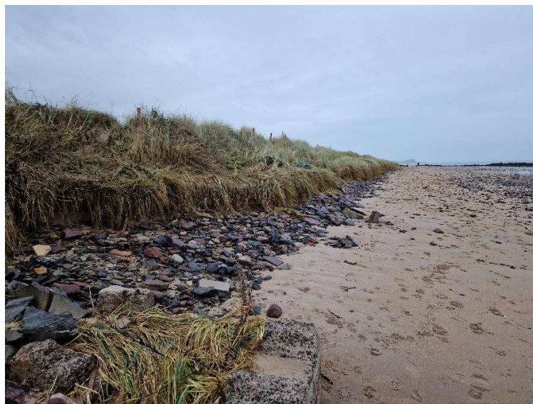
Figure 2: Burst rock-filled gabions along the 3 rd .
