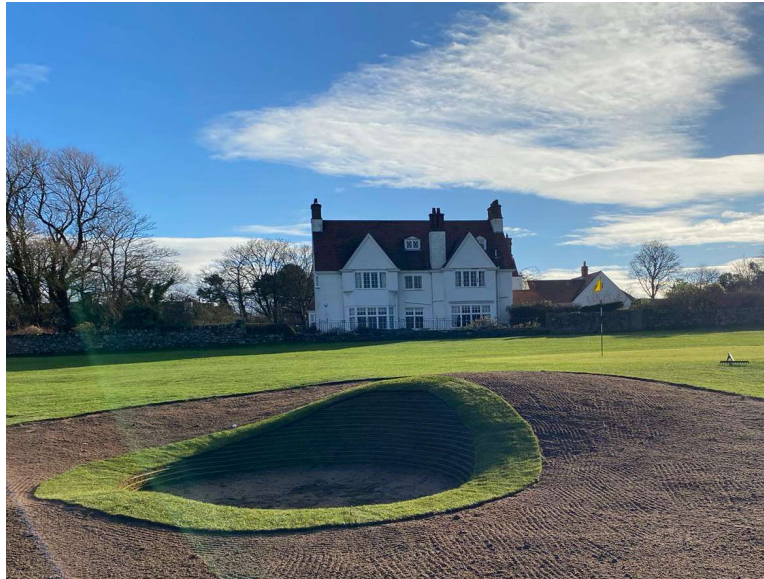
Figure 5: The rebuilt bunker was made slightly bigger and then landscaped around the sides to tie in better with the surrounds.
