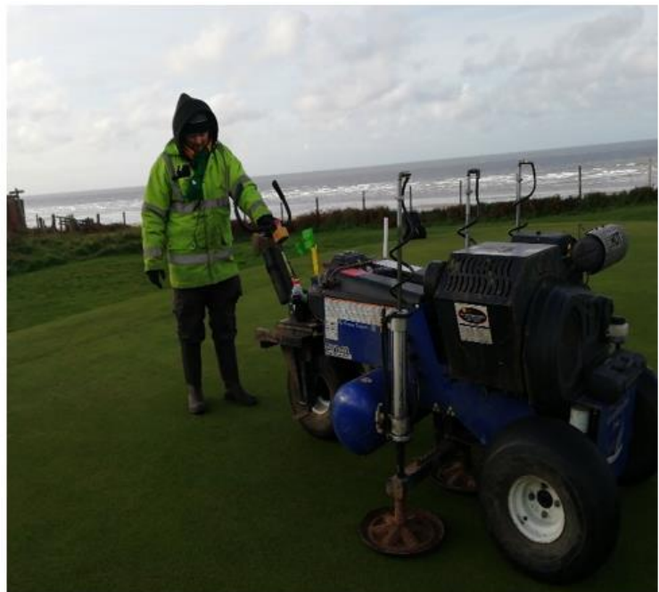
Air2G2 compressed air decompactor in operation by Richard Peel Groundworks operative on 17 th Green.
